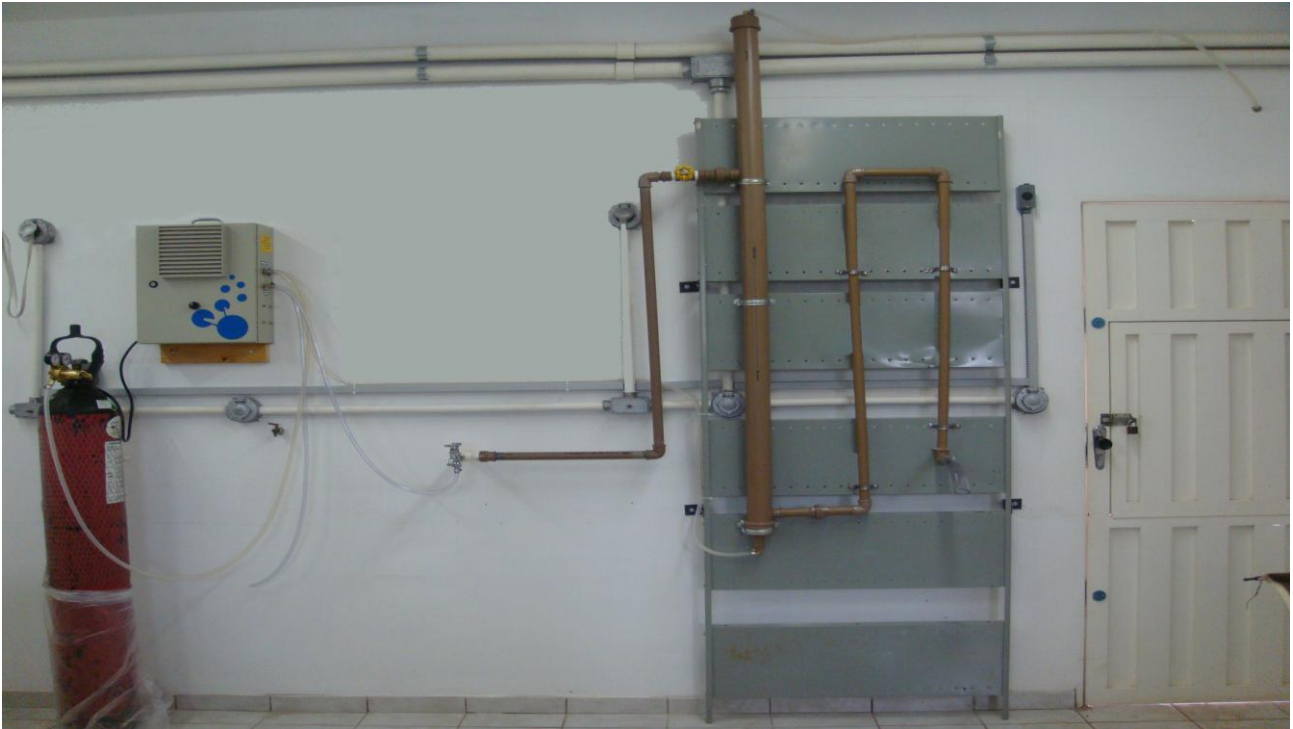
Figure 1. Equipment for production of ozonated water.
